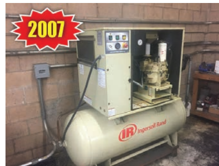
INGERSOLL RAND 15 HP ROTARY SCREW AIR COMPRESSOR
