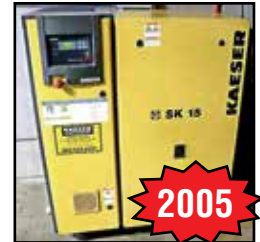
15 HP KAESER SK15 ROTARY SCREW AIR COMPRESSOR
